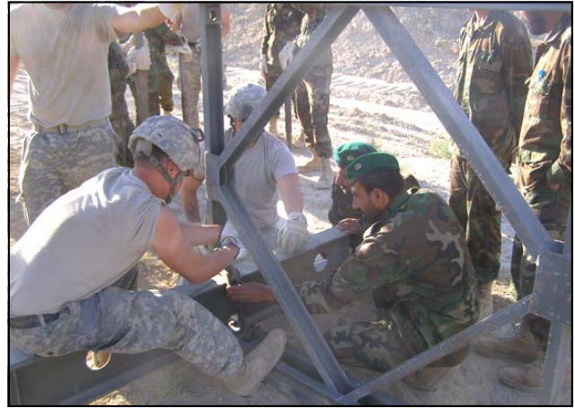
Engineer Soldiers from the Afghanistan National Army take instruction and guidance from the instructors and counterparts from 2nd Platoon, Co. C, 70th Engineer Bn. These ANA Soldiers were eager to dig and build their own bridge, and organized their own 6-man crews to lift the 600-pound panels on one side of the bridge, while 2nd Platoon Sappers built the other side.
